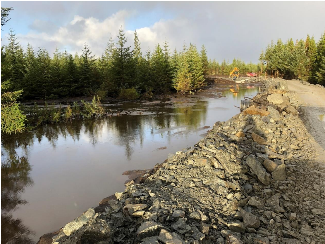
Figure 5.2 Water and sediment impoundment area upstream of Wall 1 showing stabilised situation and deposits of peat up to surface of water
