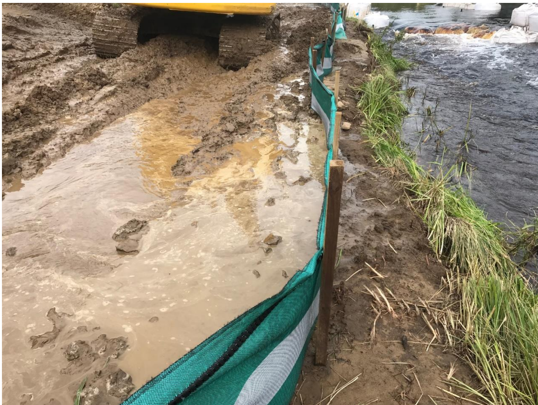
Figure 5.8 Terrastop silt fence installed on a riverbank preventing silt and soiled water reaching watercourse
