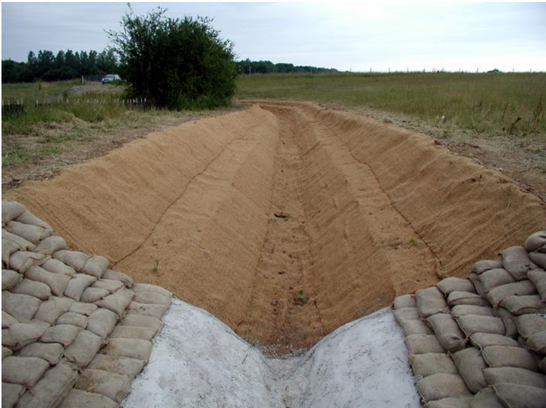
Plate 5.17 Large-scale use of CoriMesh to establish vegetated surfaces on drainage channel embankments
