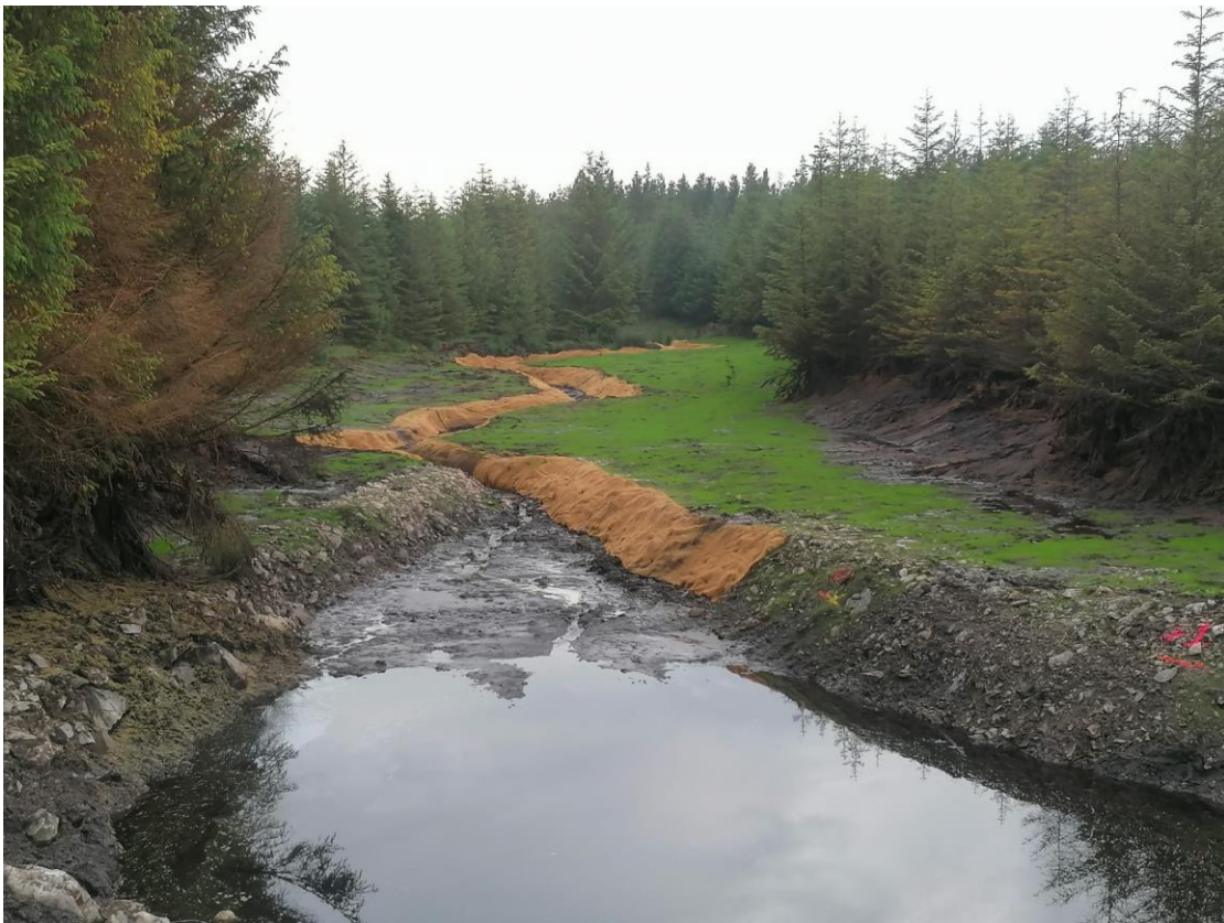
Plate 2.5 View of impounded area following sediment removal works, taken from Wall 1, facing upstream
