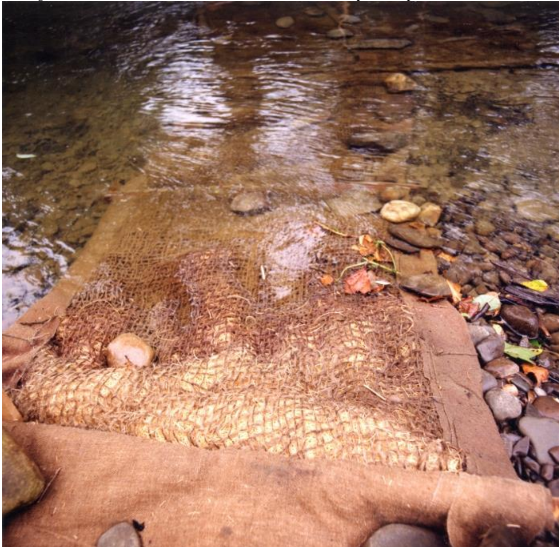
Figure 5.11 Sedimat installed on stream bed to trap suspended sediment through upper layer of jute mesh and lower layers of wood wool.
