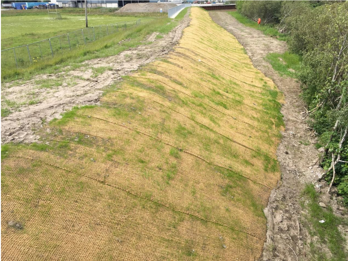
Plate 5.16 Large-scale use of CoriMesh to stabilise exposed ground, as likely required upstream of Wall 1 once large peat deposits are removed
