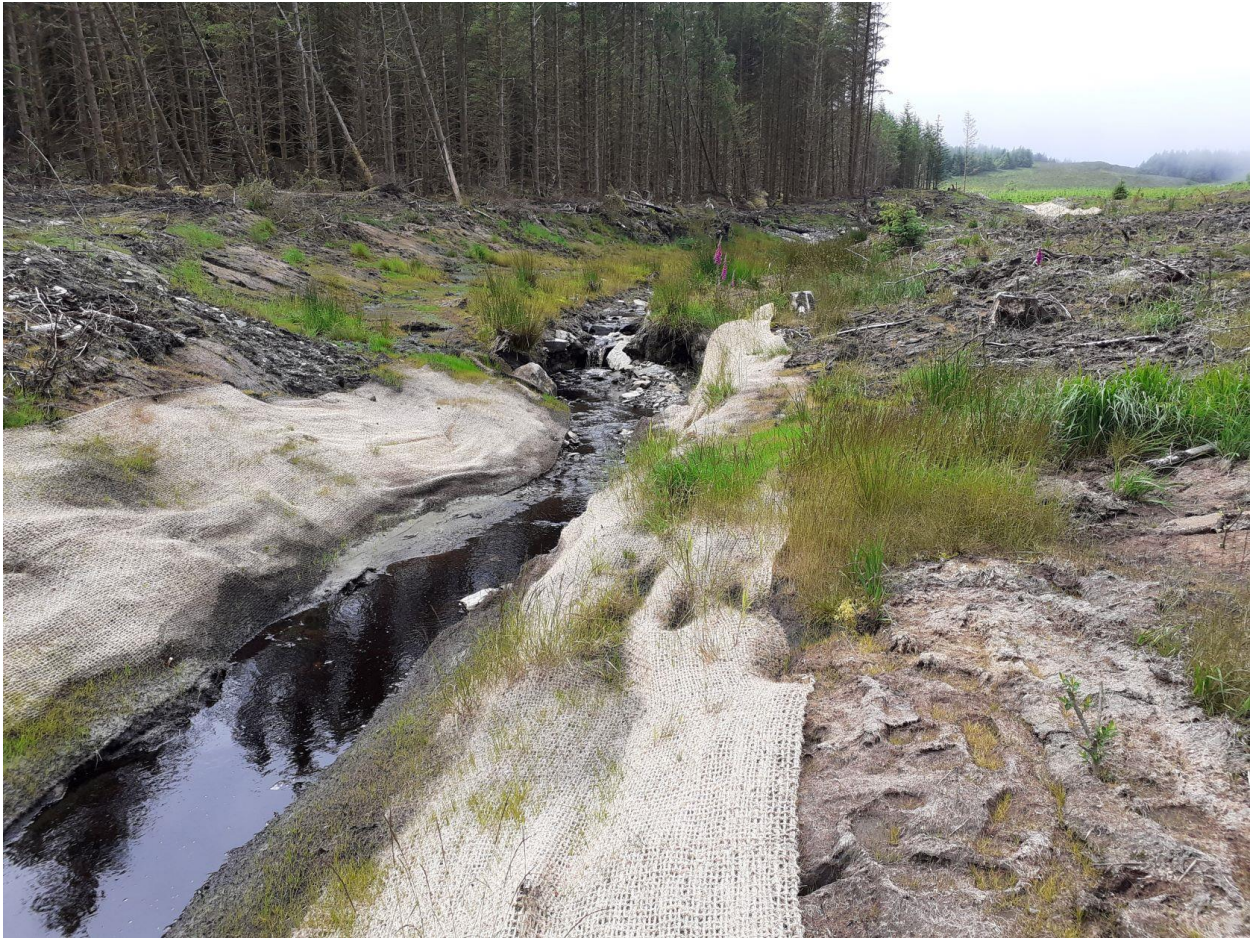
Photo 2 - area upstream of Wall 2 was located, showing grass growth in coir matting, 8/7/22
