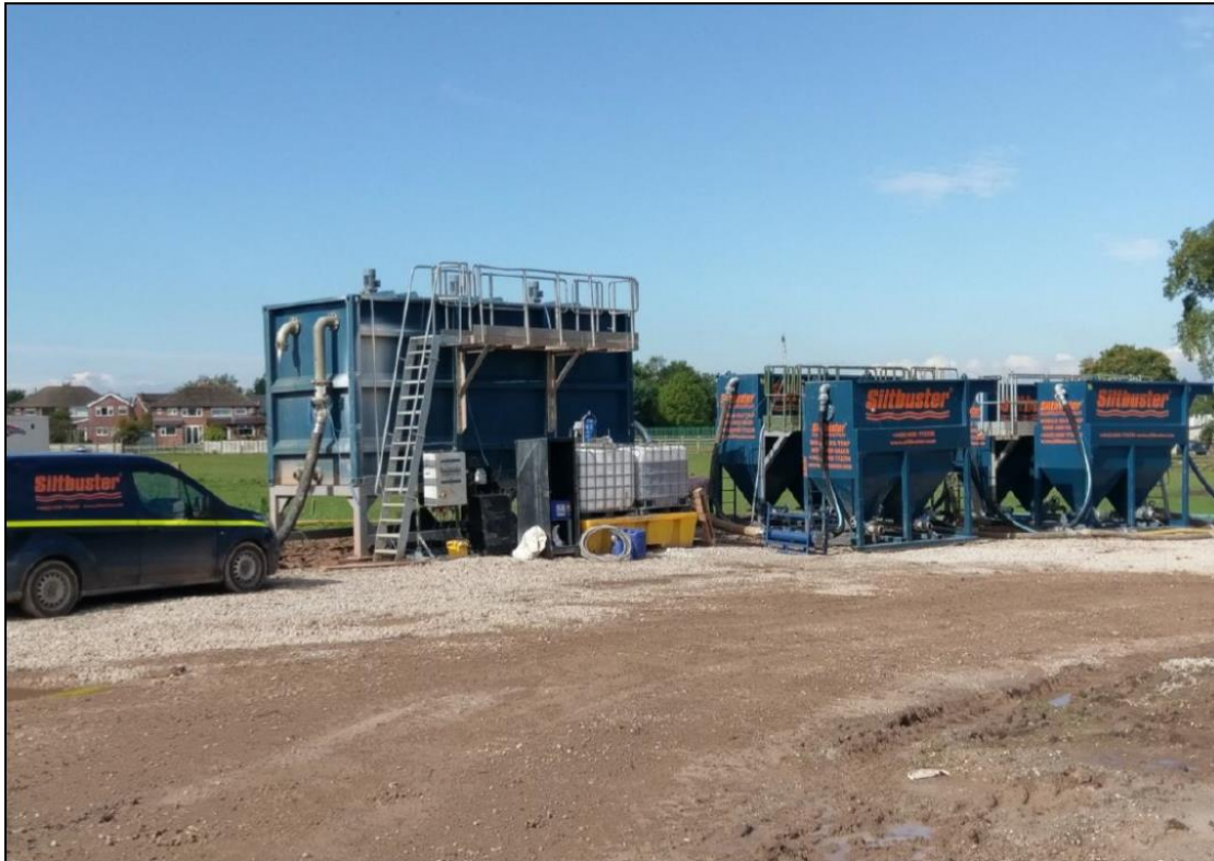
Figure 5.14: MT30 Chemical Pre-Treatment system with 4 No Lamella clarifiers
