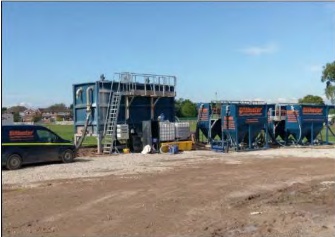
Figure 5.17: MT30 Chemical Pre-Treatment system with 4 No Lamella clarifiers
