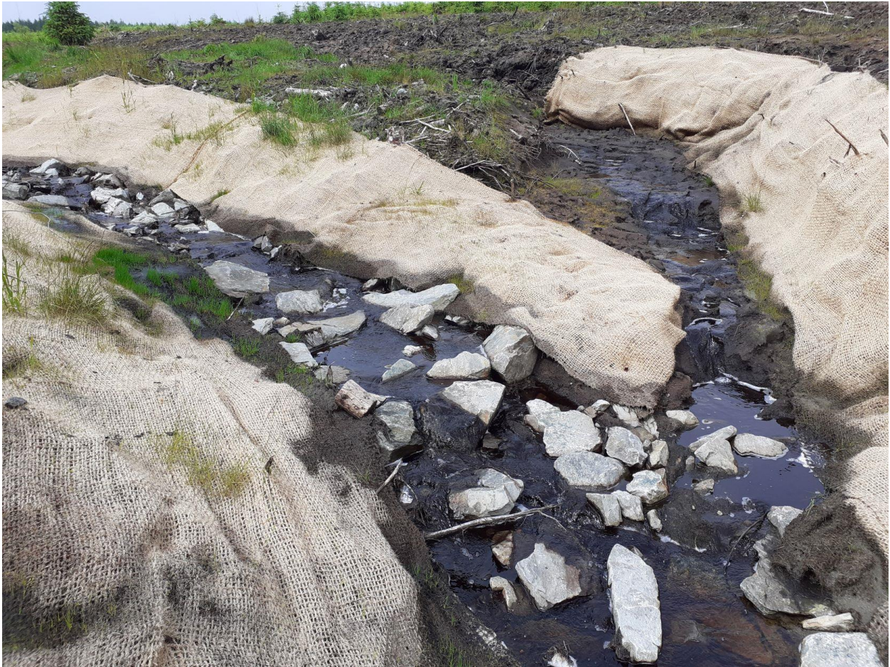
Photo 4- confluence of stream from Wall 3 & Sruhingarve stream, 8/7/22
